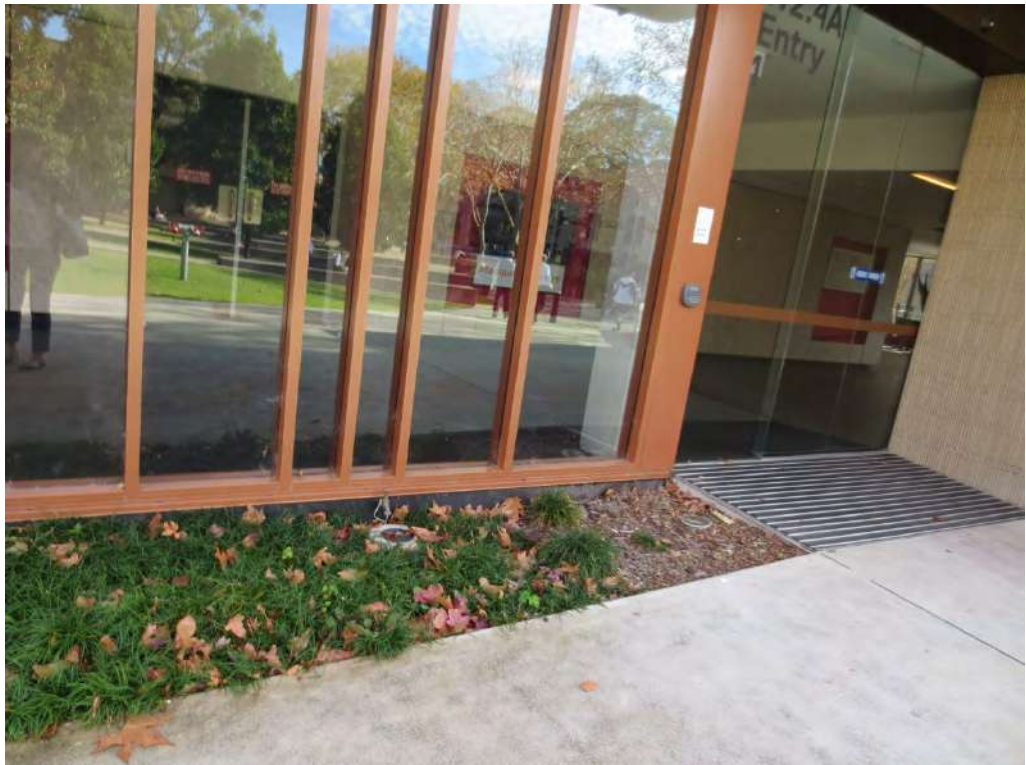
Figure 38 Mondo Grass bed requiring replacement planting
